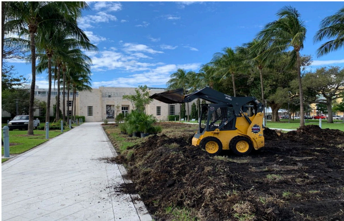
Agua dulce being installed in Collins Park in front of The Bass Museum of Art.
